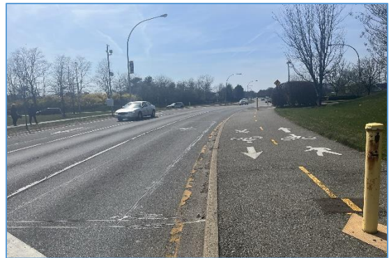
Looking east along Charles Lindbergh Boulevard, with the multi-use path on the right of the photograph.
