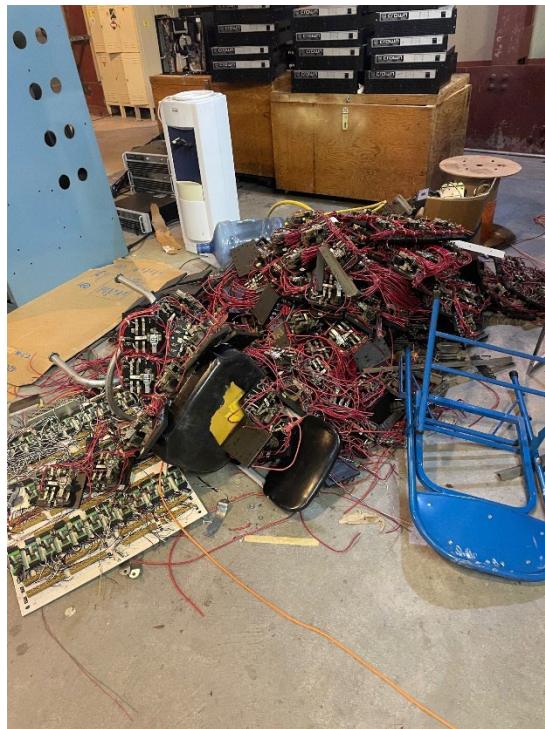
Drawing H-109 | ACM Electrical panels in Electric Room S301 at Truss Level | Date: 02-2024
