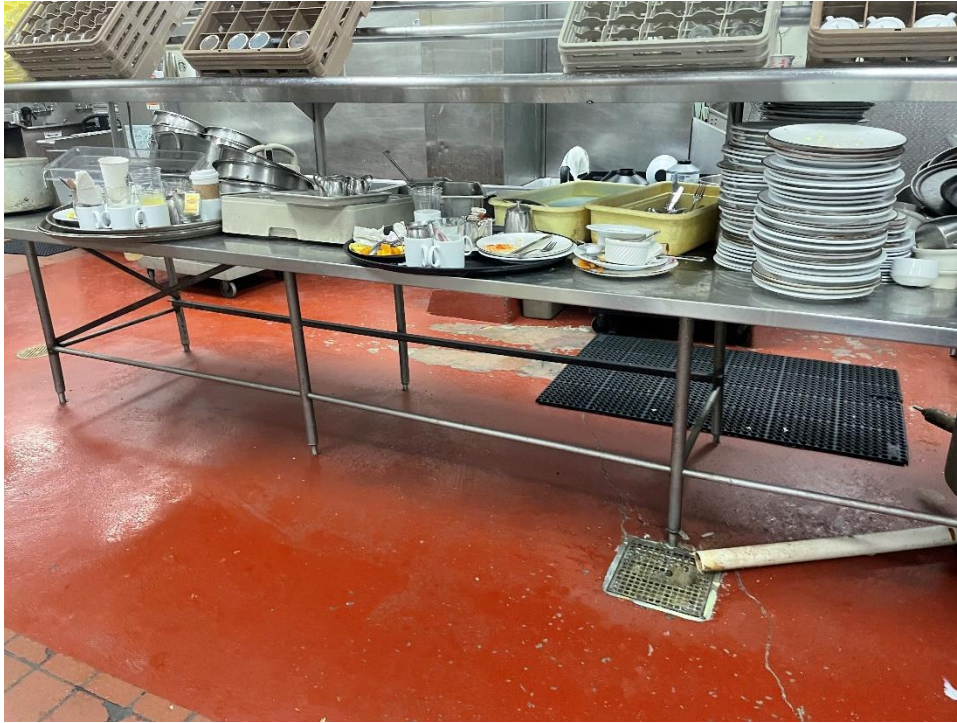
Photograph 21 – General view of first floor kitchen area and floor drain, facing west.
