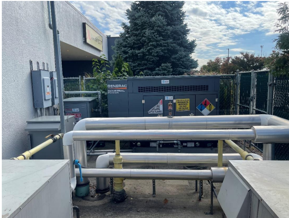
Photograph 13 – View of the emergency generator in the eastern part of the subgrade event level, facing east.
