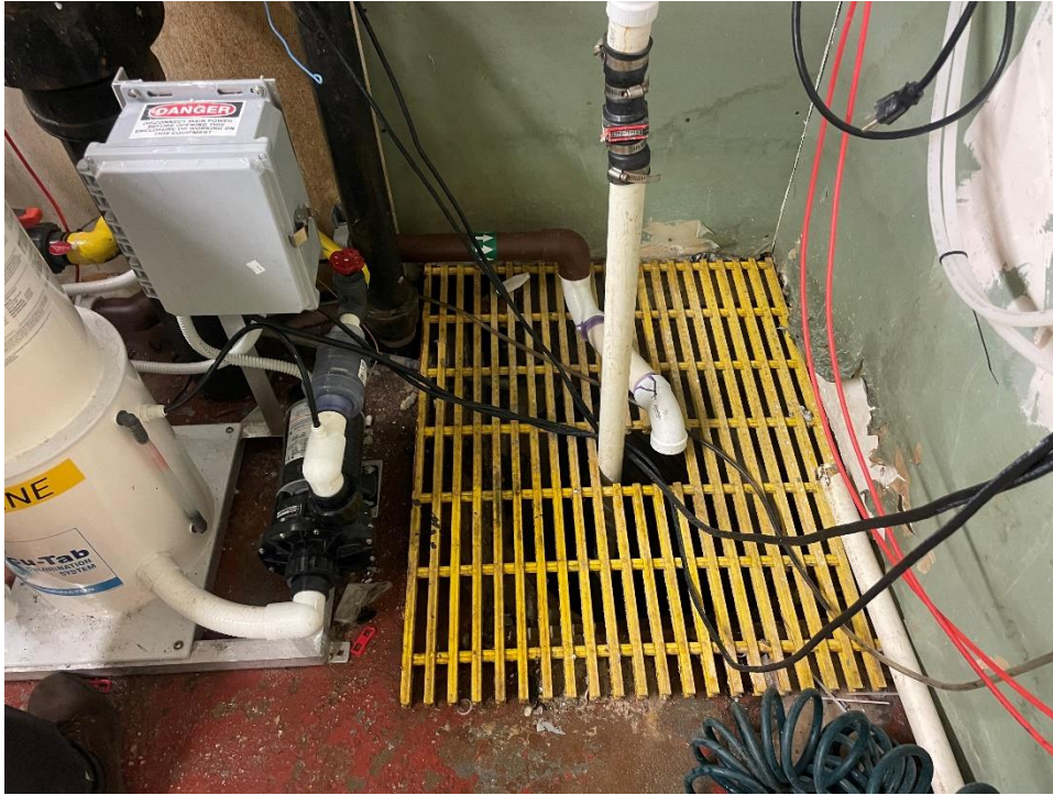
Photograph 9 – View of sump pit with pump in the subgrade simming pool area, facing north.
