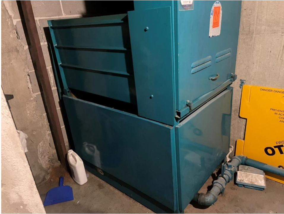
Photograph 15 – Hydraulic elevator mechanical room, southwest.
