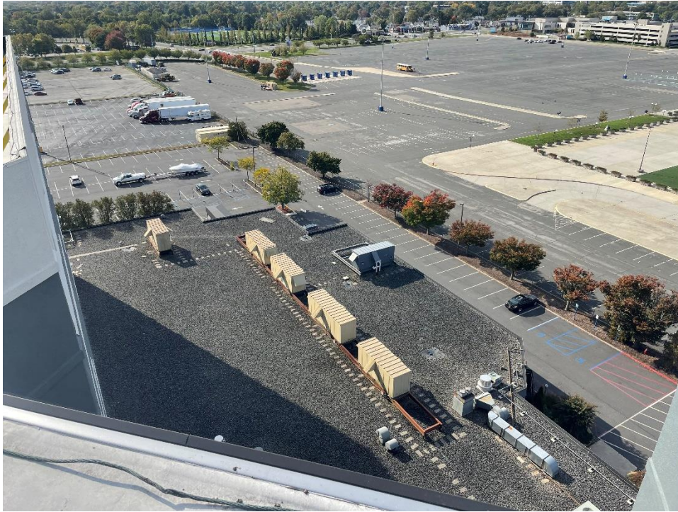
Photograph 19 – View of air handler units in the western step-out on the third-story level, facing southwest.
