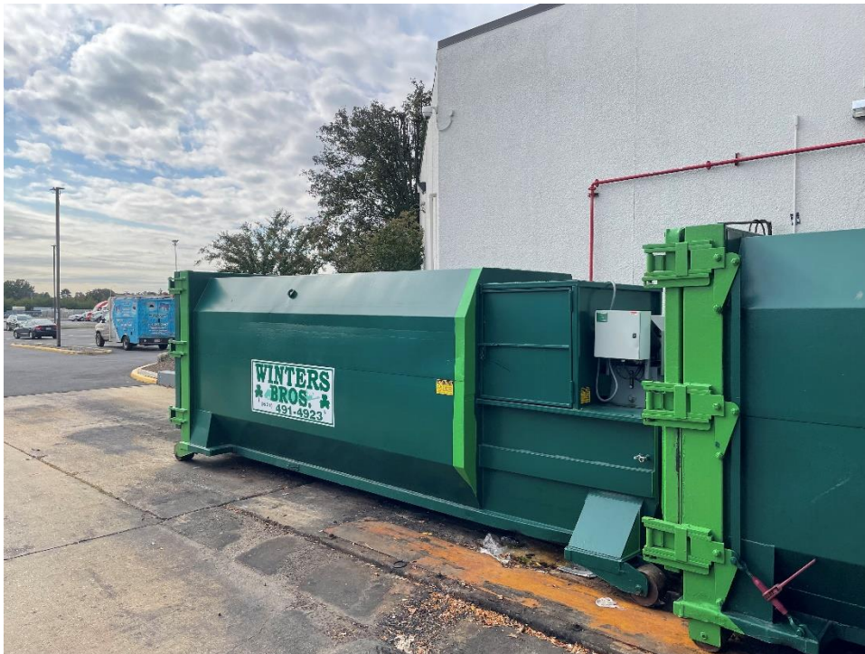
Photograph 8 – View of hydraulic compactor in the the loading dock area, facing southwest.
