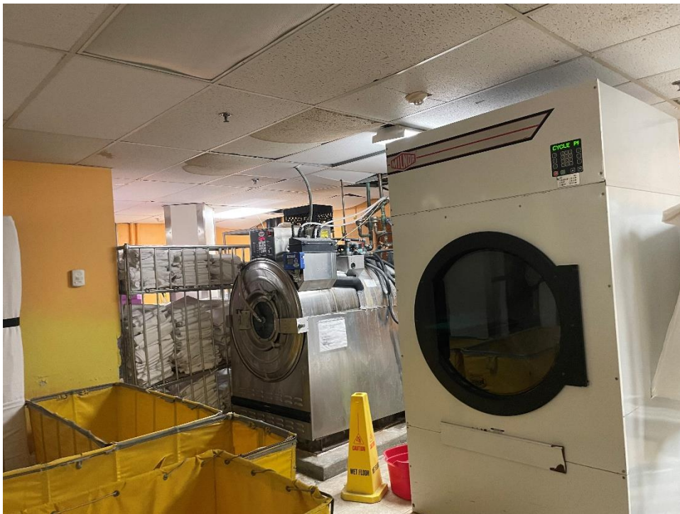
Photograph 18 – View of laundry equipment, facing southwest.
