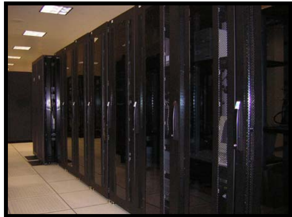
Data Center: Servers
