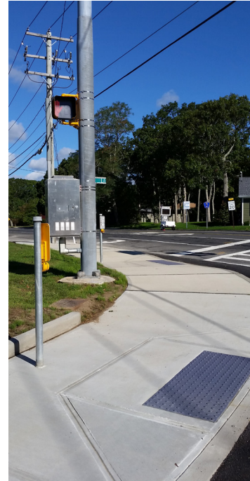
Top Left: ADA compliant pedestrian ramp with push button and new sidewalks.
