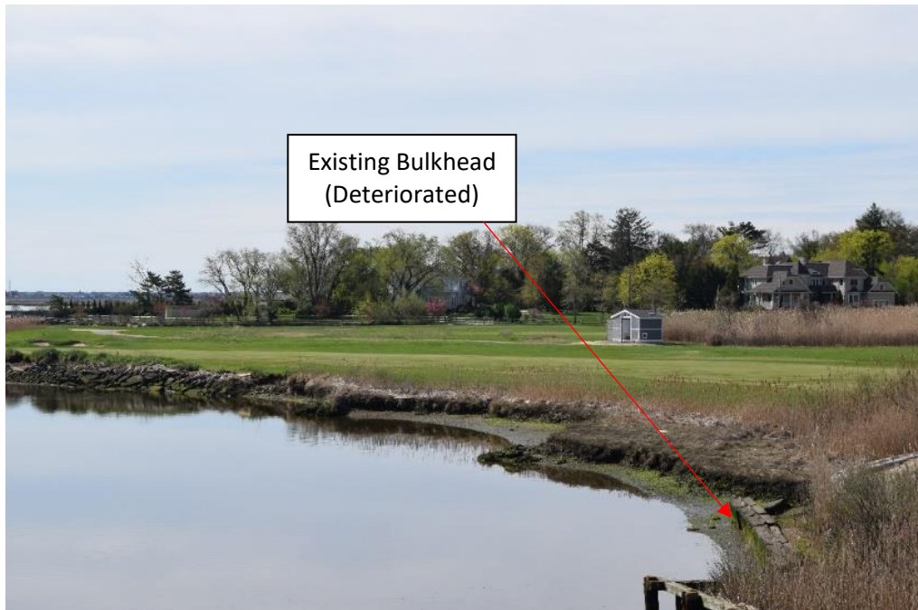
Photograph 5: Representative photograph of existing deteriorated bulkhead located along Woodmere Basin, facing southwest towards Martha Lane.
