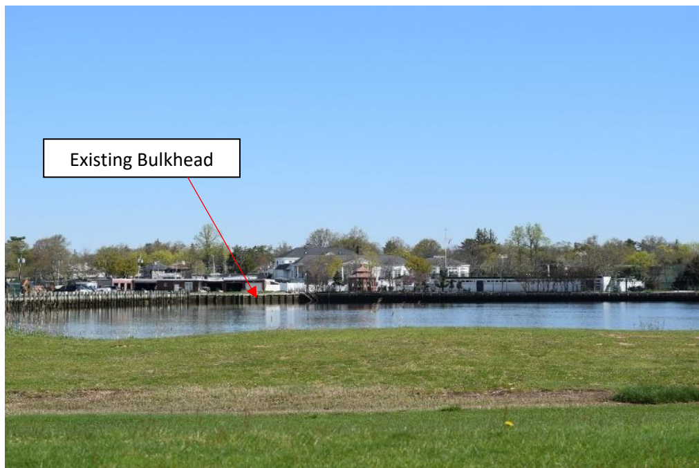
Photograph 3: Representative photograph of existing bulkhead located along Woodmere Basin, facing north towards the northwest corner of Keene Lane.
