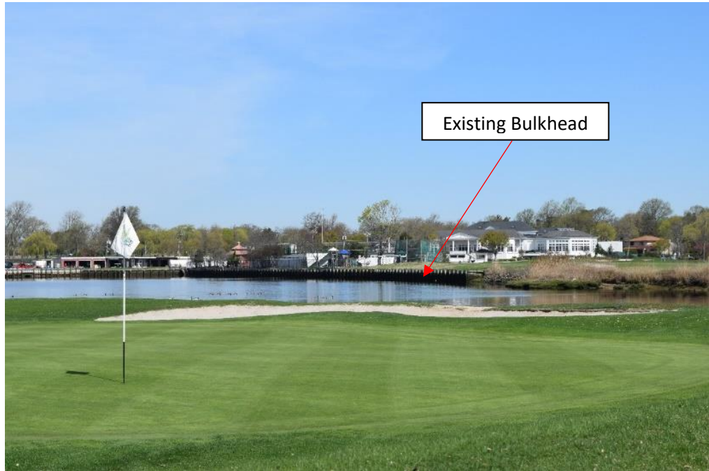
Photograph 4: Representative photograph of existing bulkhead located along Woodmere Basin, facing northwest towards the northwest corner of Keene Lane.
