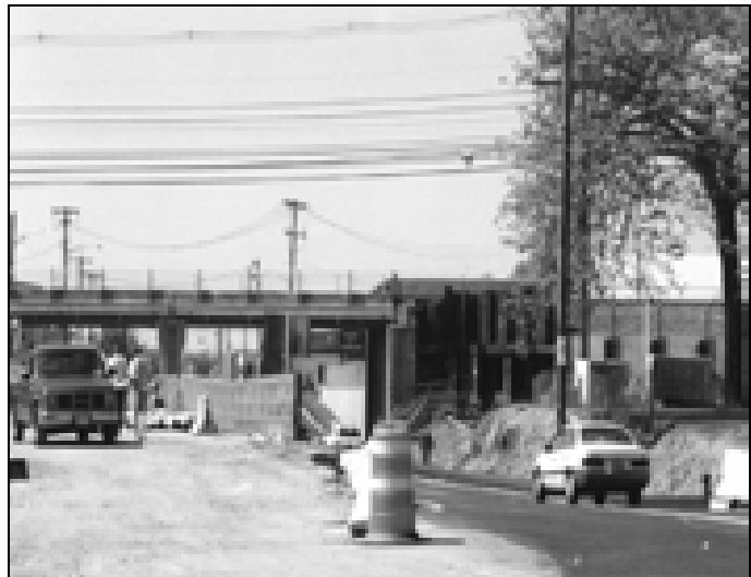
The grade crossing project in Mineola involves raising the LIRR tracks above Herricks Road.
