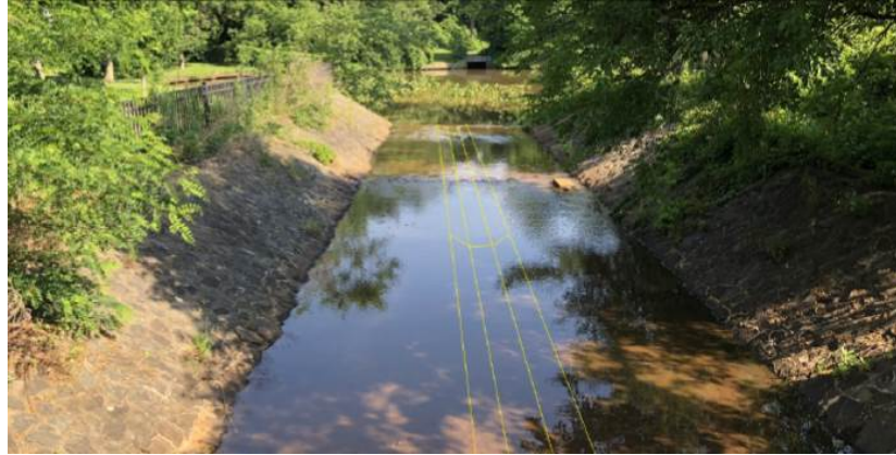
Component 4. Trapezoid Channel south of Caroline’s Pond Currently Restricting Fish Passage. Proposed Location of Low Flow Channel for Fish Passage Depicted
