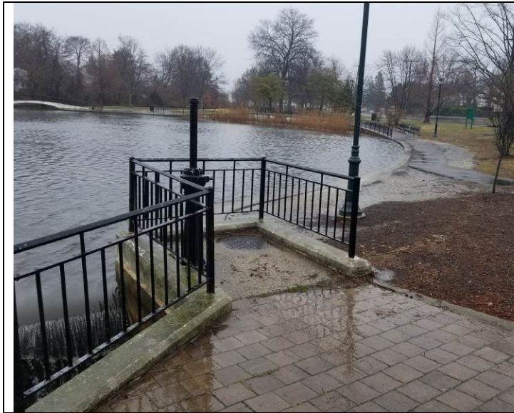
Photo 3. March 2, 2018 at Silver Lake Park east of existing weir. Flood waters have receded below the top of bulkhead elevation. Photograph taken at low tide.
