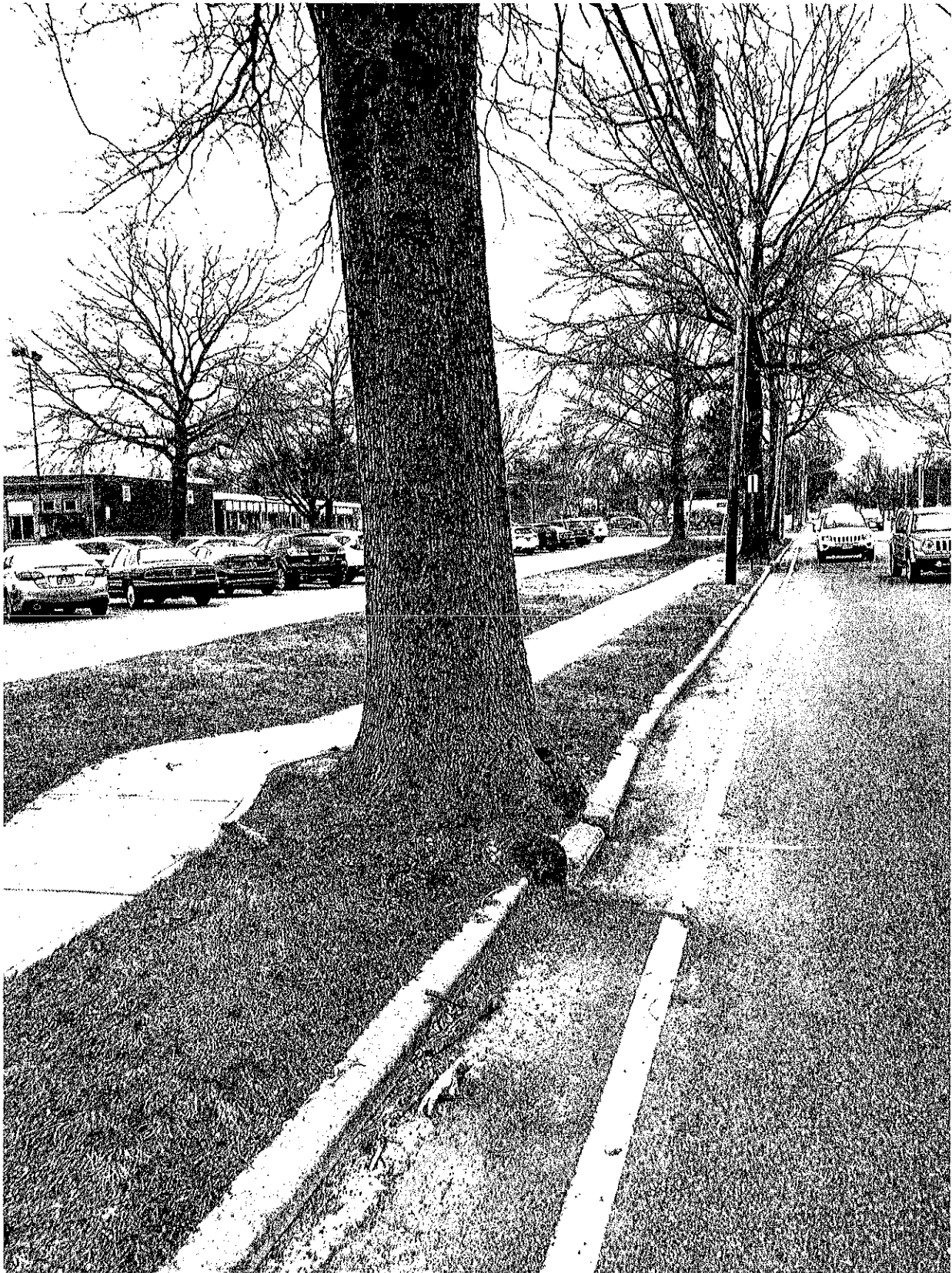
Woodbury Road Tree Removals - Example #4: Root flare pushes out curb at least 6 inches and interferes with milling. Puddling and ice slicks can occur due to improper flow of water.
