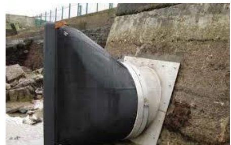
Sample Installation of external “duckbill” backflow prevention device.
