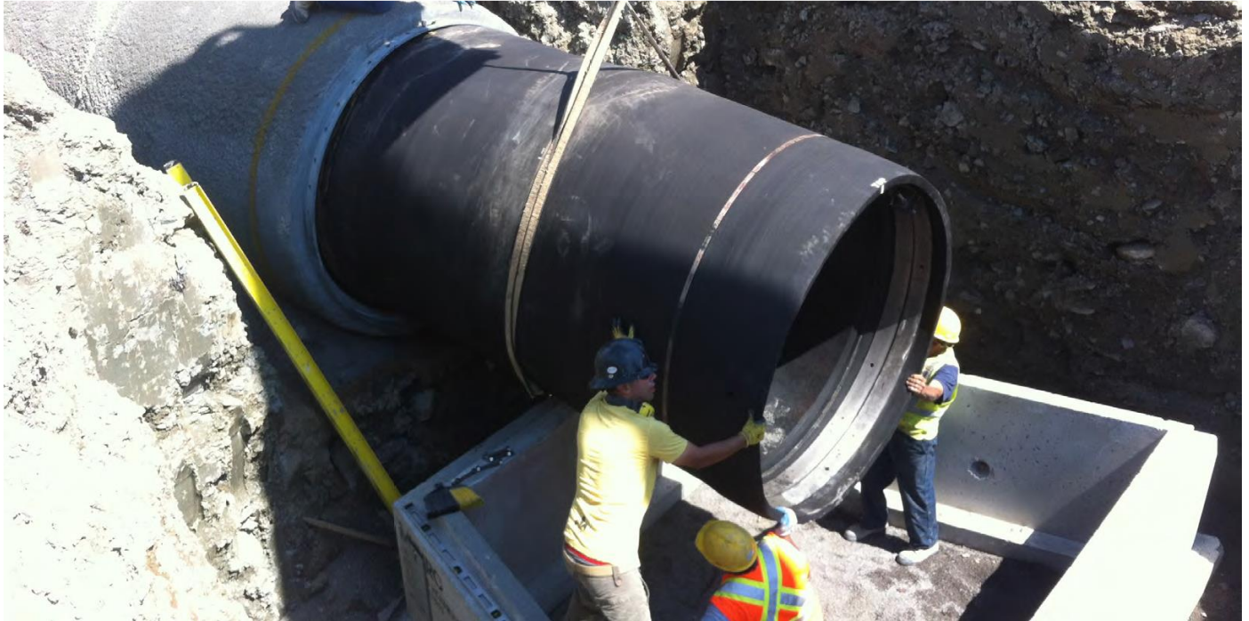
Large diameter Tideflex™ in-line check valve, being installed inside an existing drainage pipe. The existing pipe is then connected to a new access drainage structure. (Courtesy of the Red Valve Company)
