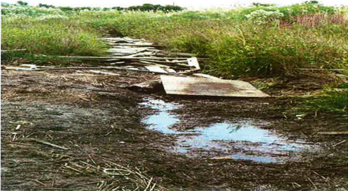
This floodwater ditch, filled with sand and debris, is in need of maintenance to prevent mosquito breeding.
