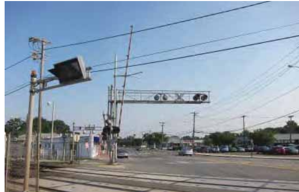
The conditions at the intersection of Railroad Avenue and Stewart Avenue make for a dangerous crossing.
